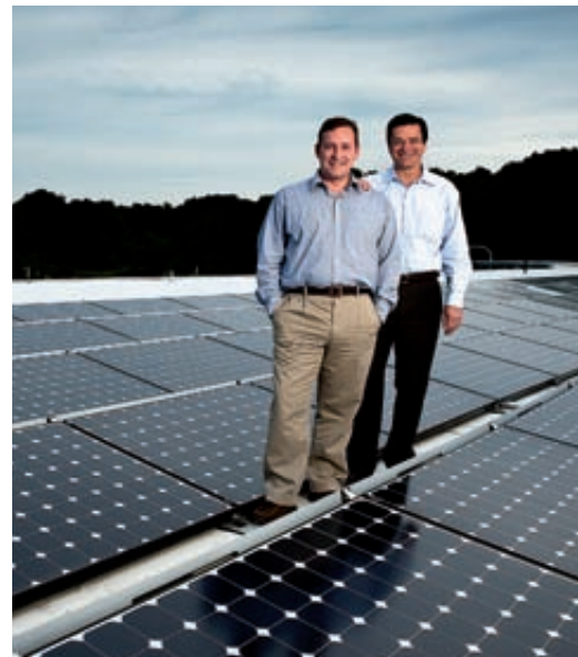
SOLAR: 20,000 sq ft of solar panels at National Grid's New England corporate office
